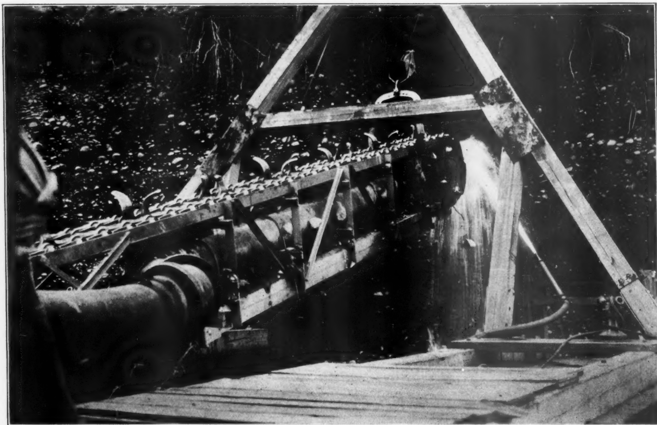
Suction Line Showing Flexible Suction Hose Connection
